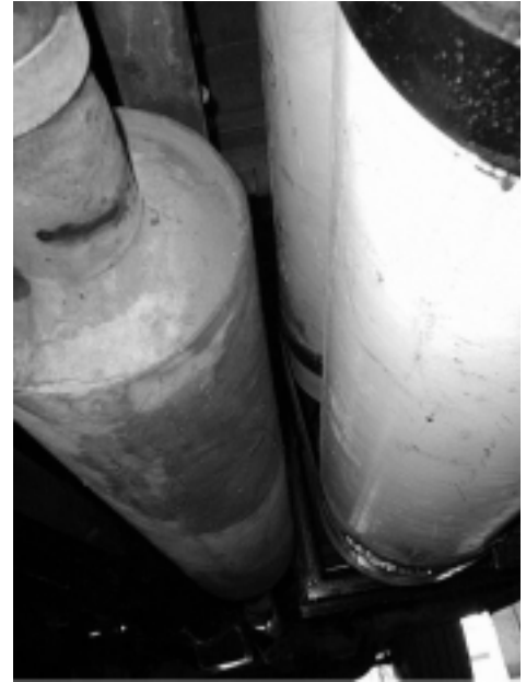
Figure 4: CNG cylinder on converted bus, less than 2 cm from exhaust muffler
