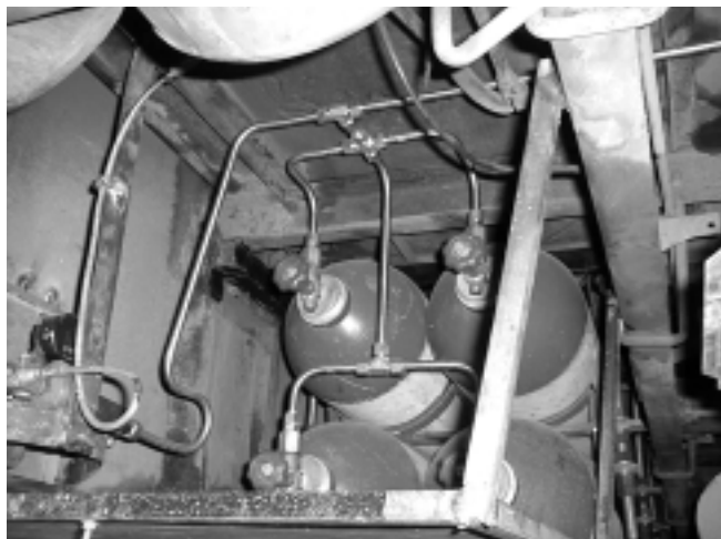
Figure 3: CNG piping on a converted bus, \frac{1}{2} inch diameter without stress relief loops, inadequate clamping of gas pipes
